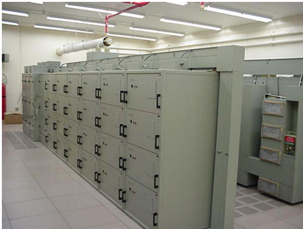
Figure 6: Loran Station George's 48 HCG Transmitter
